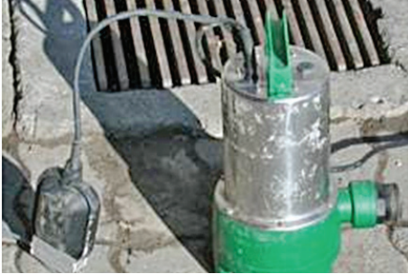
Photo 15: pompe de relevage (AGRIDEA).
